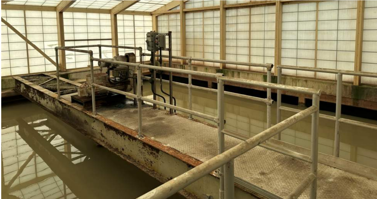
Figure 2.4 Detritor Building (ventilated to the OCS-2111 Carbon Unit) with Noticeable Signs of Corrosion, likely due to H 2 S.
