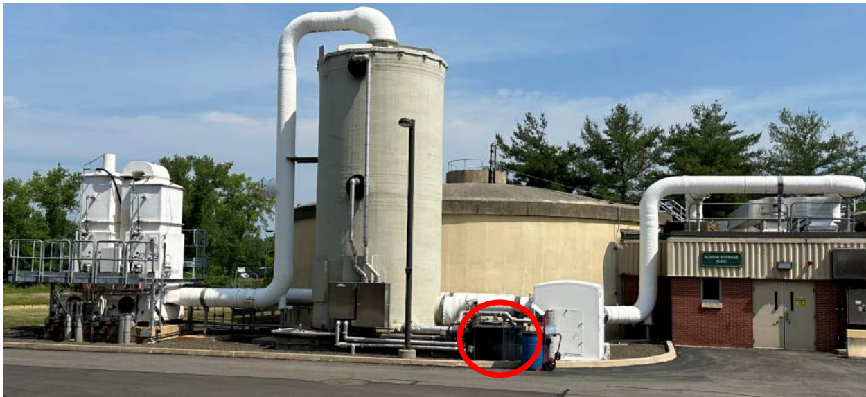
Figure 2.1 Sludge Storage Tanks OCS-2131 BTF-Wet Scrubber Odor Control Unit with Signs of Corrosion on the Base of the Wet Scrubber Stage
