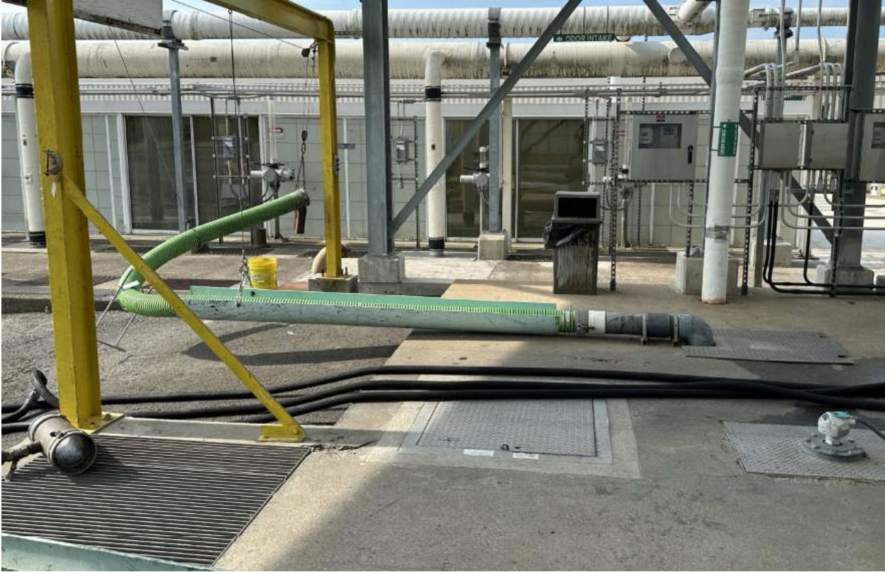
Figure 2.5 Septage and Sludge Receiving Station Ventilated to the OCS-2113 Carbon Unit
