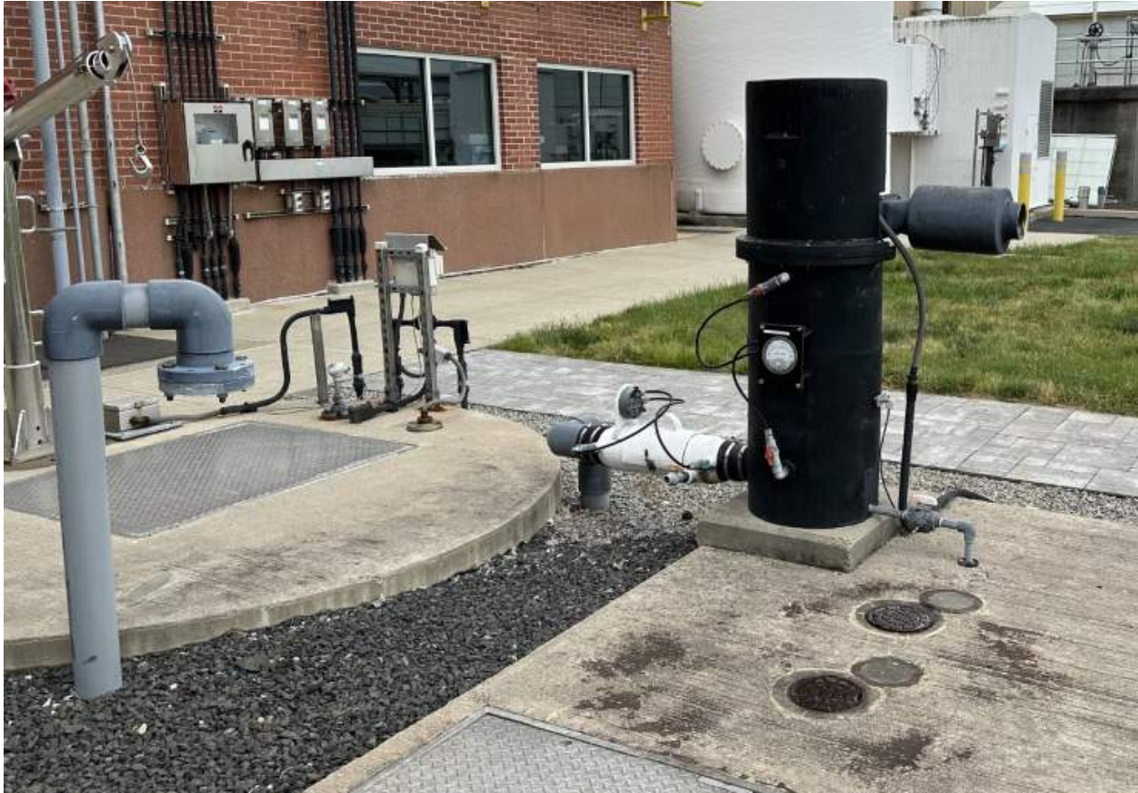
Figure 2.3 Centrate OCS-2117 Carbon Unit
