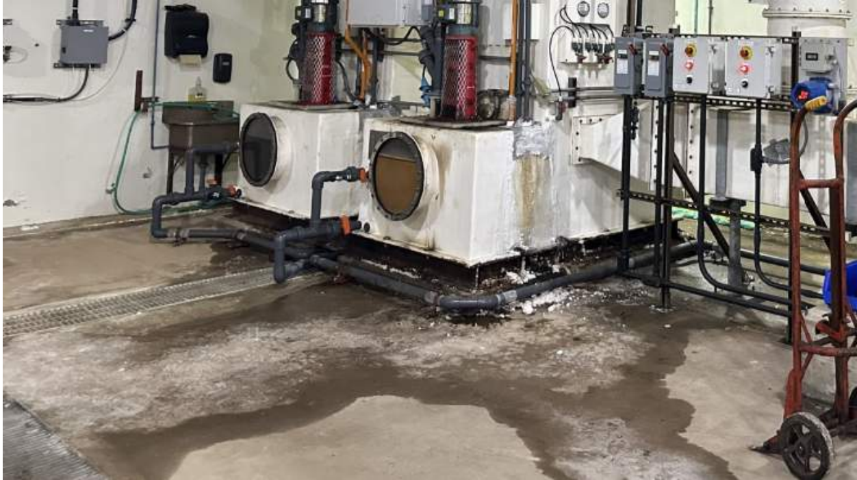
Figure 2.2 Dewatered Process Wet Scrubber OCS-2121 Odor Control Unit with Major Signs of Corrosion, Prominent Deterioration of the FRP Vessel, and Chemical Spills
